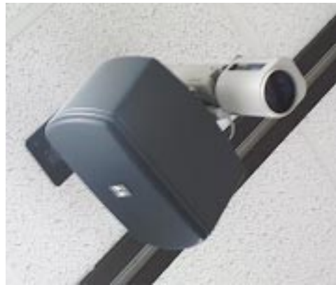
Ceiling mounted overhead camera and room speaker
